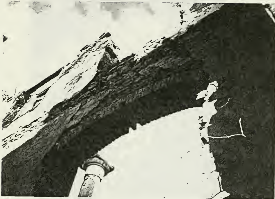
Figure 27: Southernmost arched opening along east elevation, showing loss of stucco and missing bricks within the arch itself
